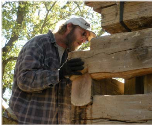
Eric Sammons, log specialist, works to insert replacement log on the Rice house near Dalton.
