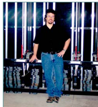
Kelly Grooms stands in front of the "Fly System" located backstage. This sophisticated technological design houses the rigging equipment used to raise, lower, or move from side to side the scenery, the lights and the actors.
